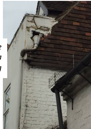
Maintenance issues on a listed building
