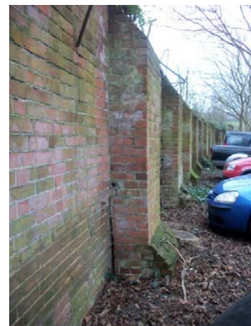
Vulnerable brick boundary wall to Caversham Court allotments on The Warren
